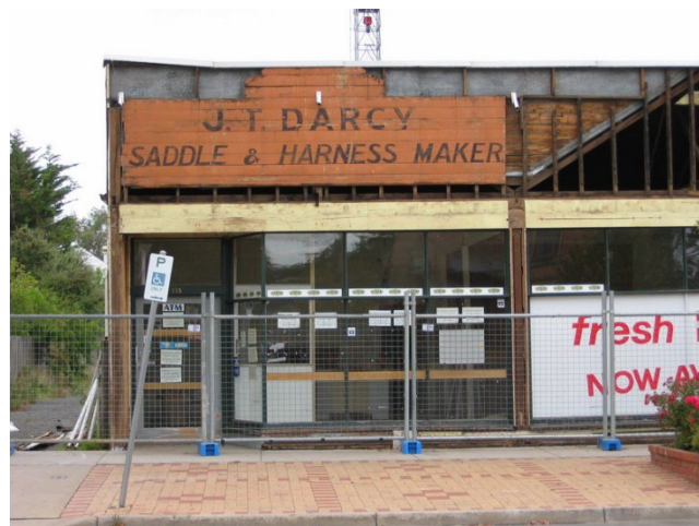
Photo 2: Early remnant parapet of J.T. Darcy's saddle and harness making shop during demolition, 2005.
