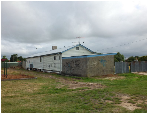
Photo 11: Rear (west) and south elevations of Ballan Bowling Clubhouse showing skillion addition of concrete block construction, 2015.
