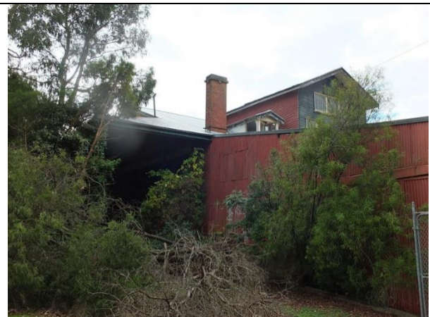
Photo 6: Former Butter Factory, south elevation, 2014. The left portion is the porte-cochere of 1908, with original chimney and small lantern light. The elevated gabled wing is the addition of the 1930s.
