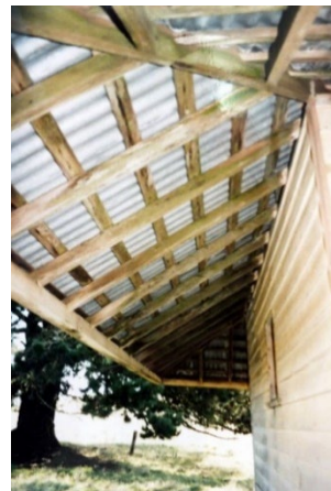
Photo 4: Former 'The Pines' dairy, eaves detail, n.d. [c.1990s]. Source: June Huggins, Ballan.
