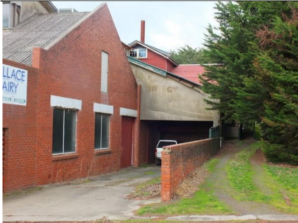
Photo 3: Former Butter Factory (Building 1), north elevation, west end, 2014. The front wing (left) is the addition of the 1940-50s, the gable end behind (with concrete infill) is the addition of 1922 and the attic gable is the addition of 1928.
